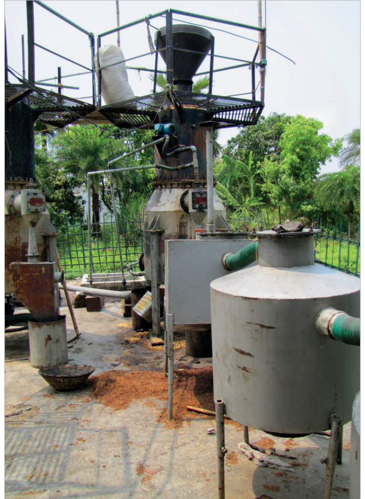
New Delhi, India: Energy generating plants powered by risk husk waste.
